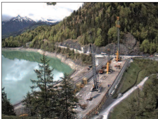
(a) View of the cut-off construction with the grabs and hydro-cutters on the crest of the Sylvenstein dam in the summer of 2012; downstream, widening of the dam crest with an angular retaining wall. The reservoir water level is lowered by about 5 m. This is a view from the webcam of the State Office for Water Management [Wasserwirtschaftsamt Weilheim, 2015 8 ].
