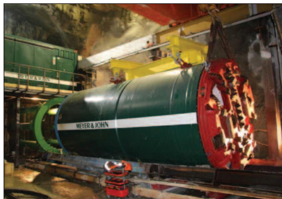
(c) Installation of the TBM. Behind it: the thrust unit station with six hydraulic cylinders for 2500 t thrust, and above that, the driving control station.
