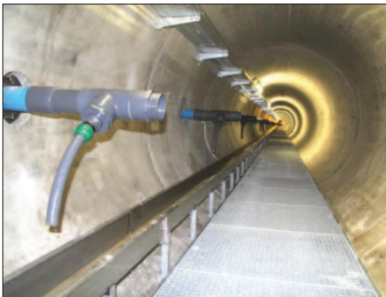
(g) View of the control gallery, the seepage control system and the interior fitting.
