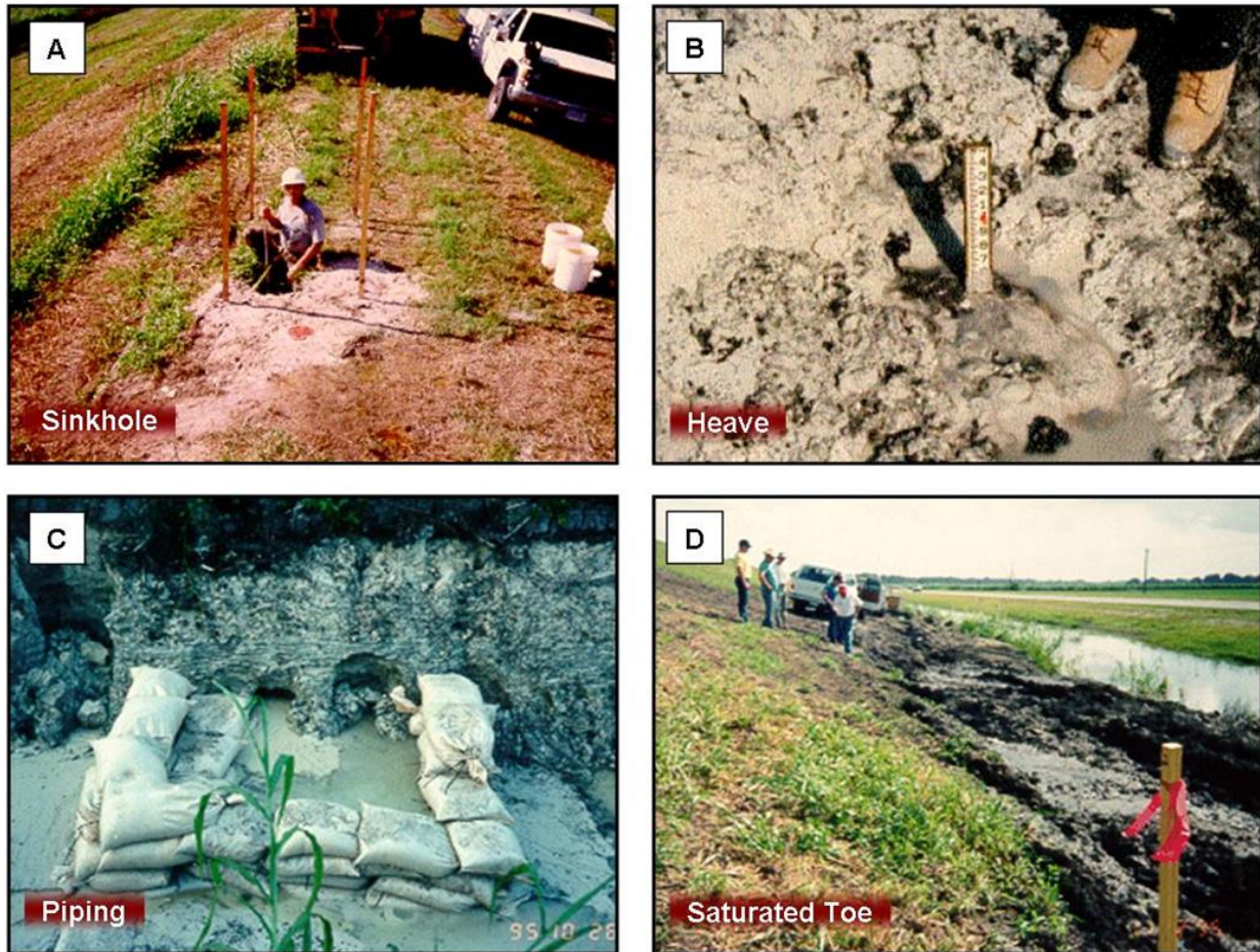
Figure 1: Types of observed dike damage: (A) Sinkhole formation in crest, (B) heave of downstream toe, (C) piping at downstream toe of dike, and (D) saturated soils at the ground surface of landward toe (Toe Ditch in Fig. 2) and embankment slope (from Davis et al. 2009).
