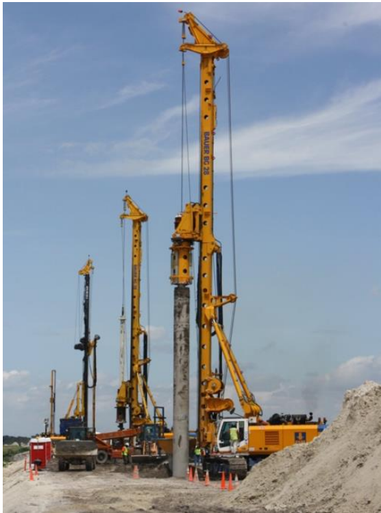
Figure 3: Two BAUER BG28 rigs (in front) drilling replacement columns (Arnold et al. 2011).
